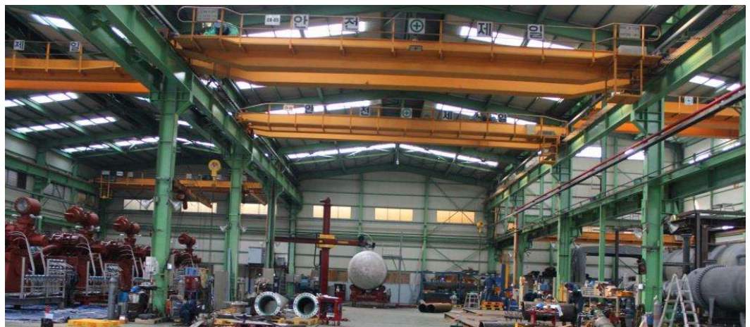
Overhead Crane (30T, 10T, 5T)
